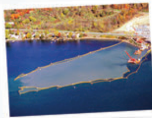
Turbidity barriers restrict the flow of silt laden runoff from a land disturbance, confine it to a limited area, and allow the silt and sediment to be collected.
