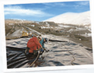
This tailings dam liner in Siberia was installed during the winter months to limit environmental impacts on the local hydrogeology and to keep the mine development on schedule.
