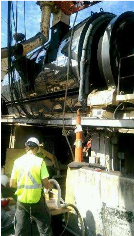
The Line-Vac® is used to transport ACE Fiber™ to the RAP Collar at a Drum Plant
