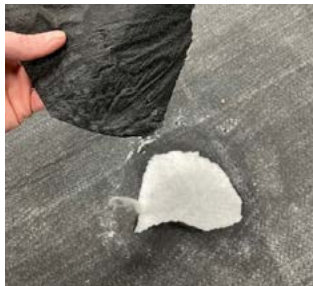
Figure 1: Damaged conductive layer.
